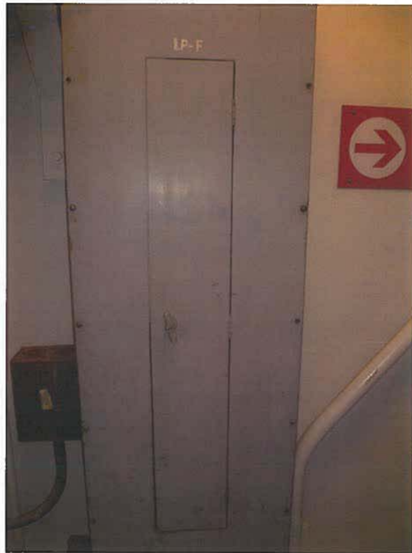
EXISTING PANEL "LP-F"
