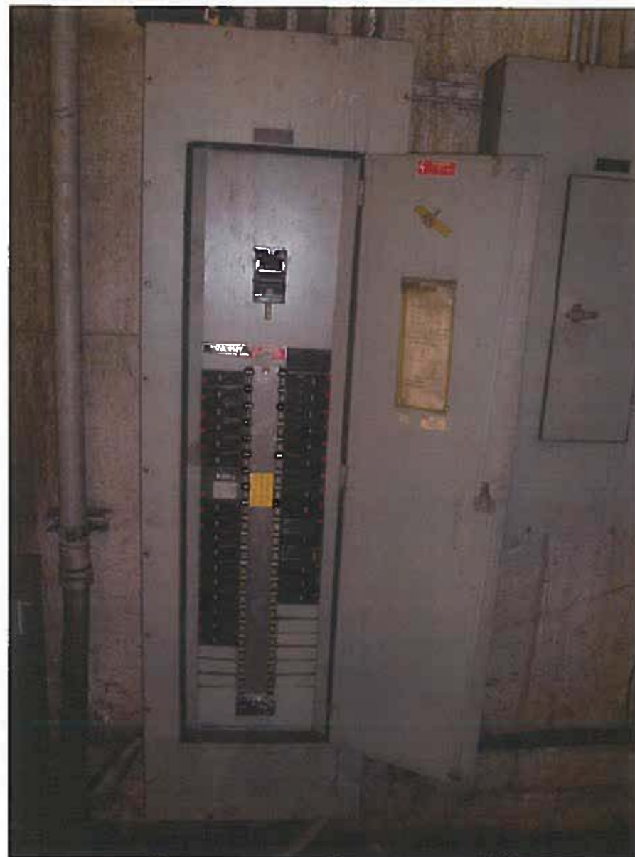
EXISTING PANEL "MSAA"
