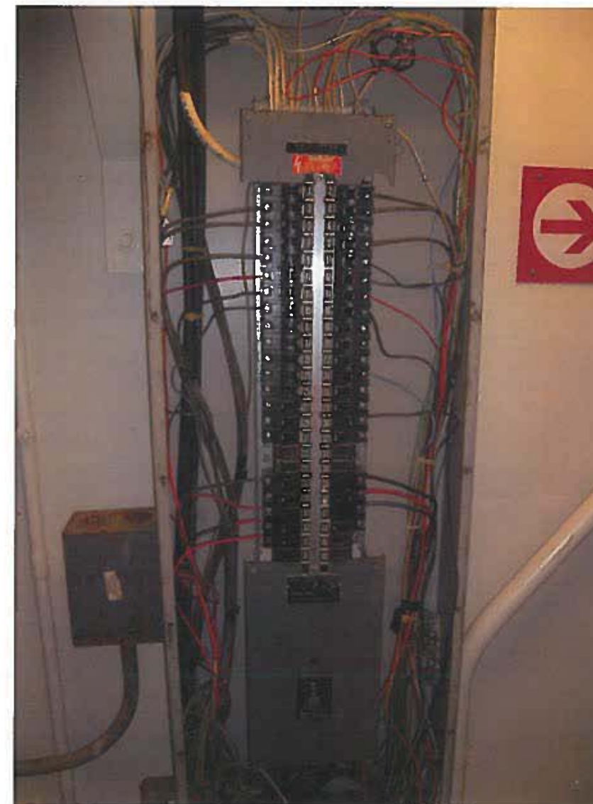
EXISTING PANEL "LP-F"
