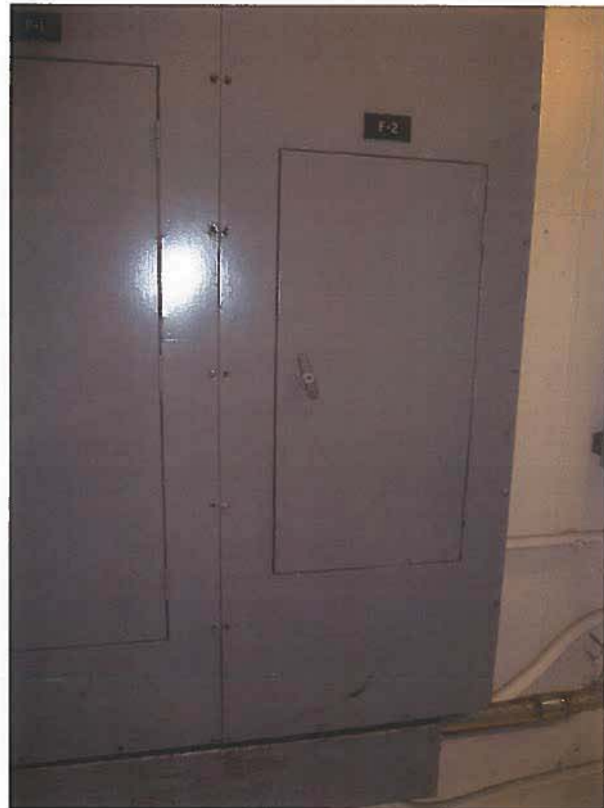
EXISTING PANEL "F-2"
