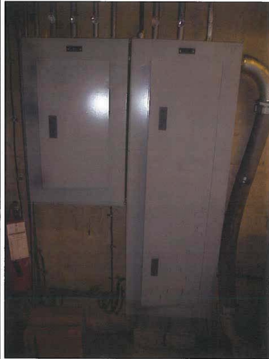
EXISTING PANEL "F1"
