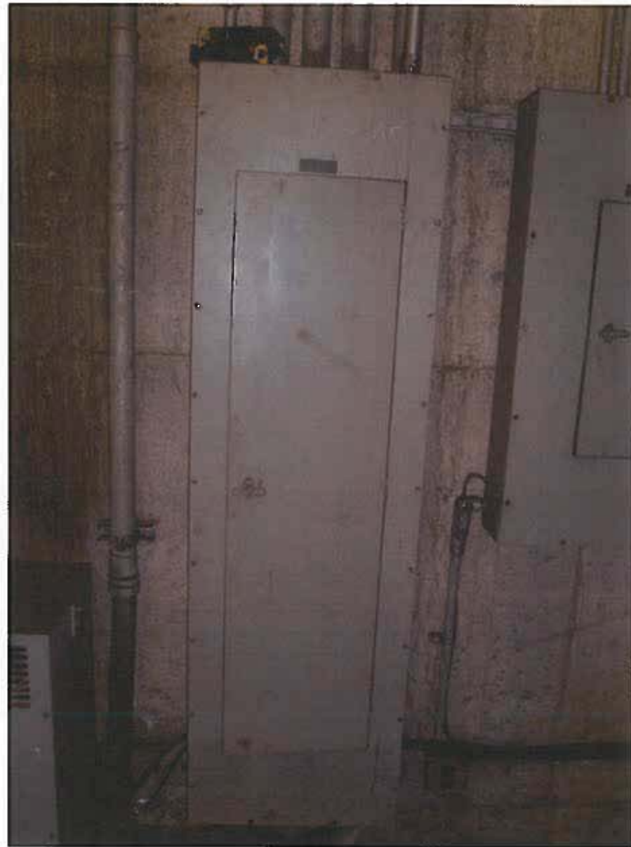
EXISTING PANEL "MSAA"
