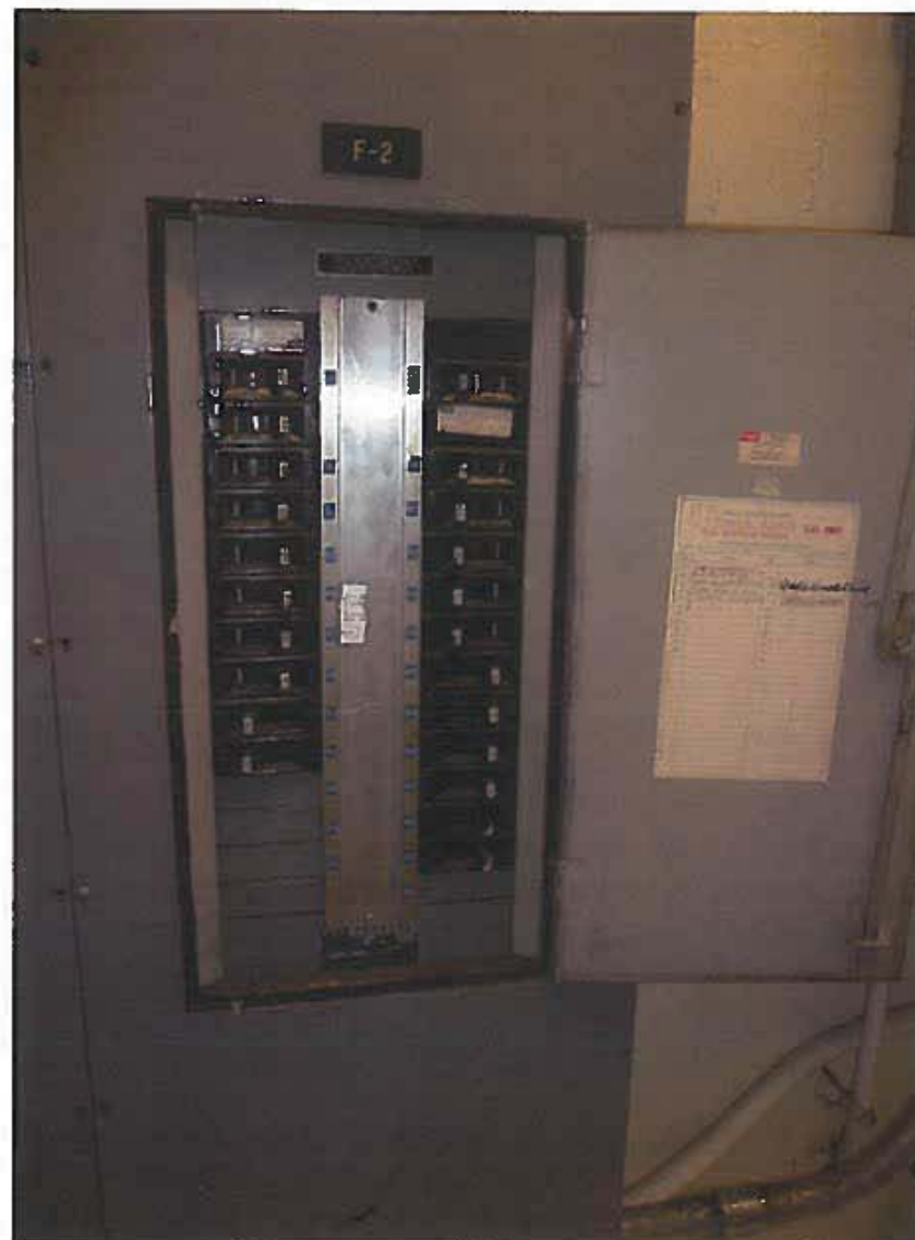
EXISTING PANEL "F-2"
