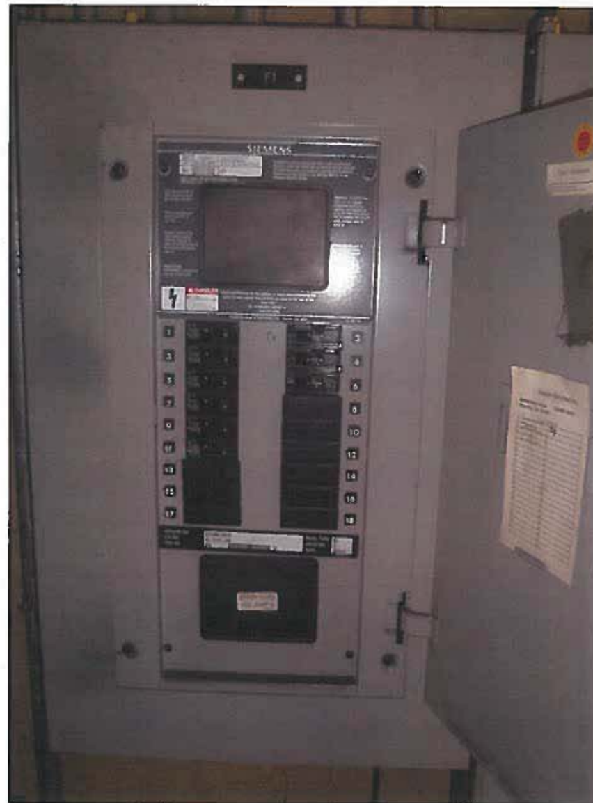
EXISTING PANEL "F1"
