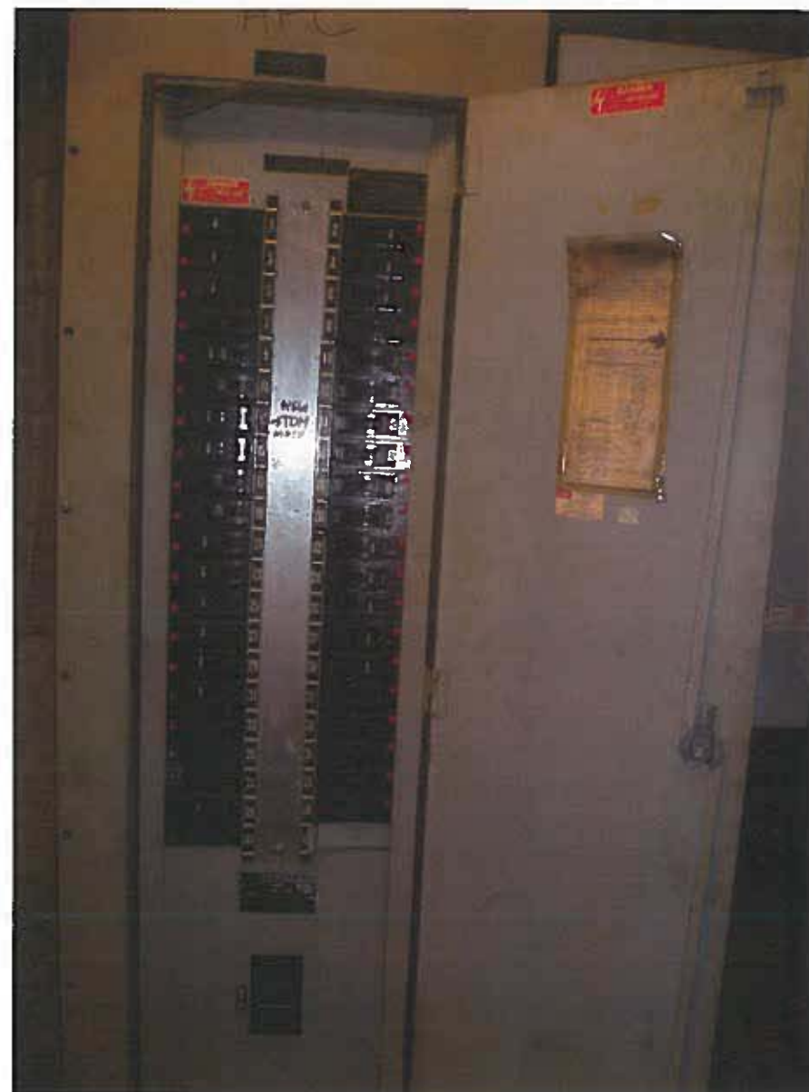
EXISTING PANEL "MNCC"
