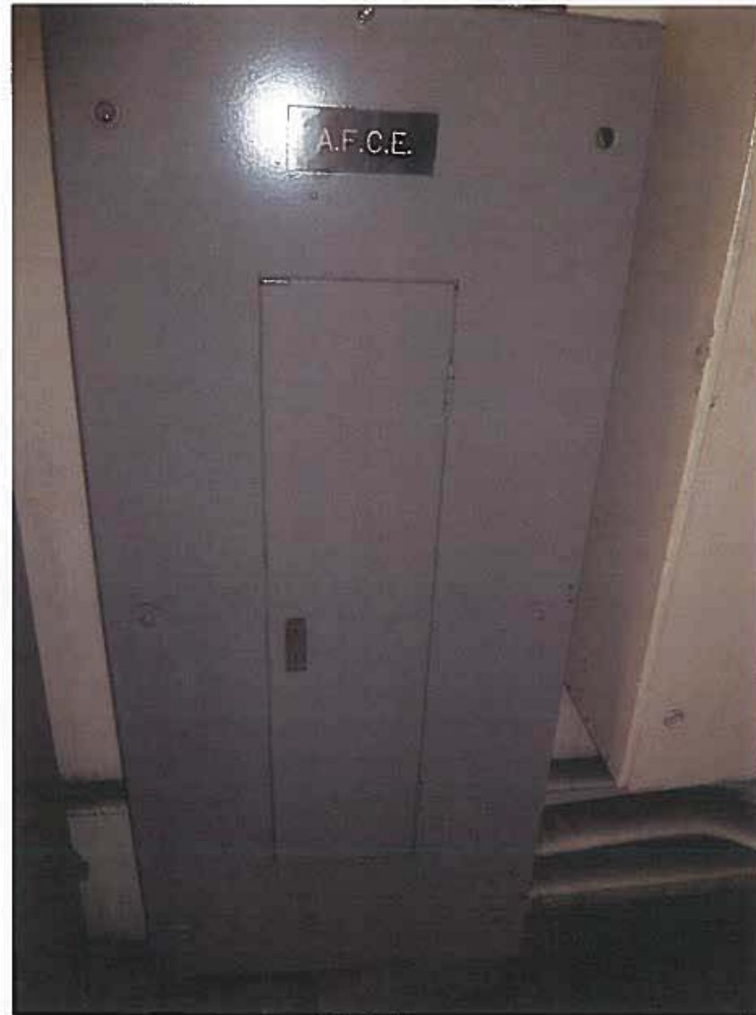
EXISTING PANEL "AFCE"
