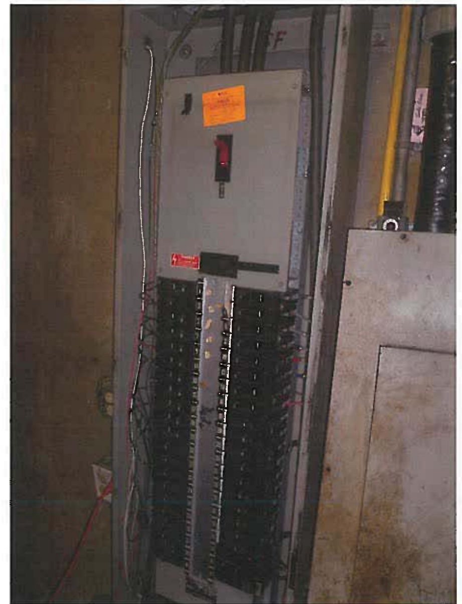
EXISTING PANEL "SF"
