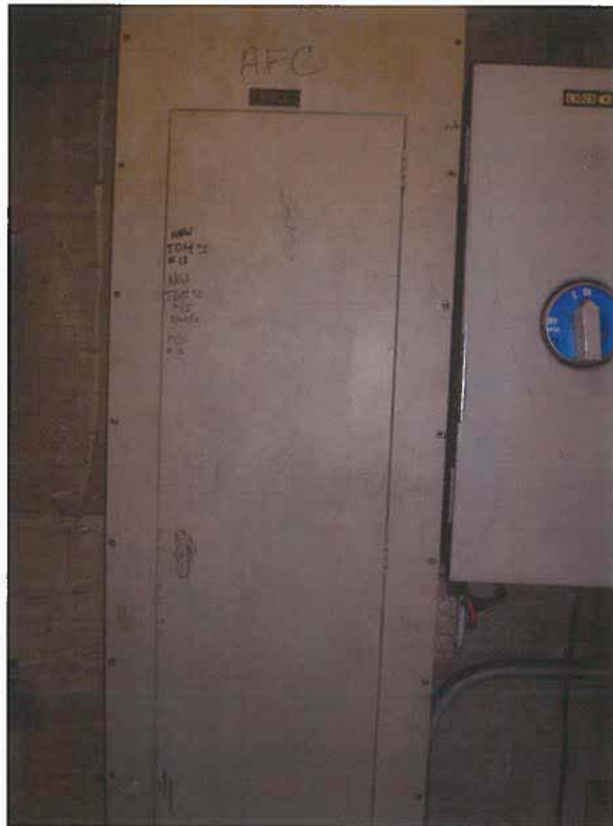
EXISTING PANEL "MNCC"
