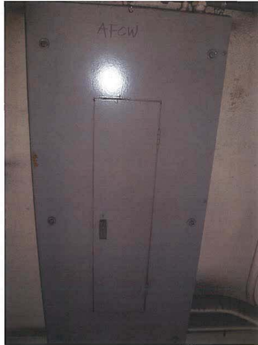
EXISTING PANEL "AFCW"
