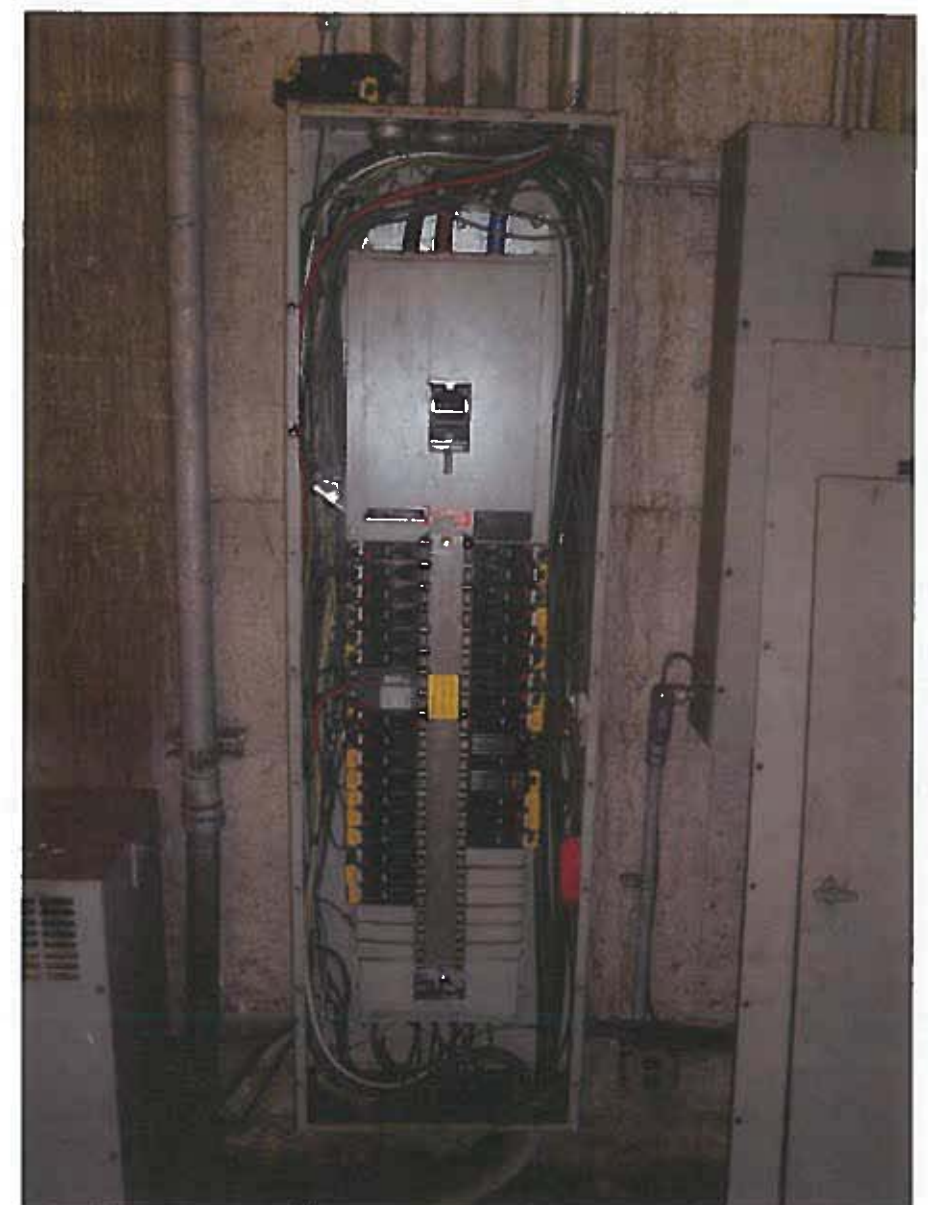
EXISTING PANEL "MSAA"
