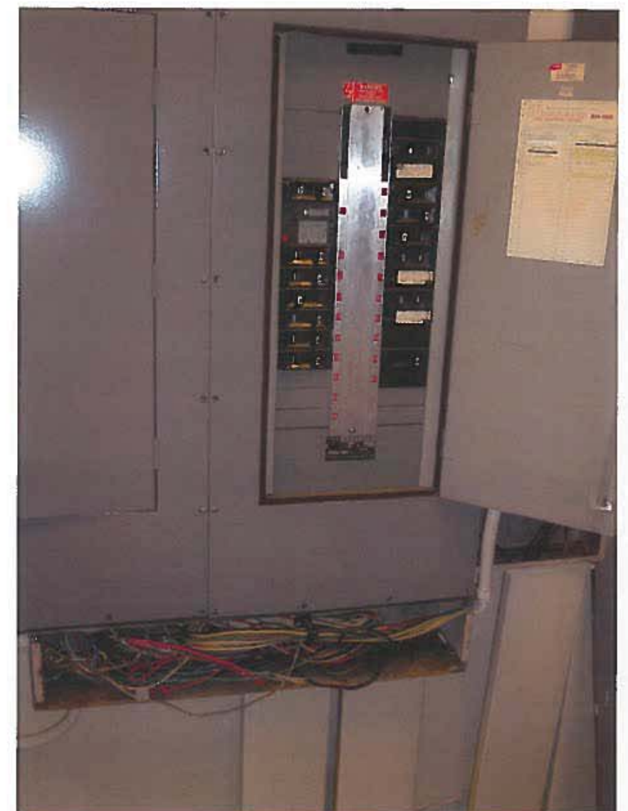
EXISTING PANEL "NMF-2"
