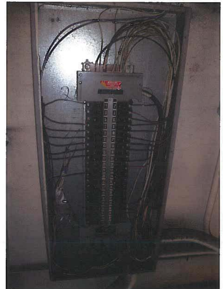
EXISTING PANEL "AFCW"
