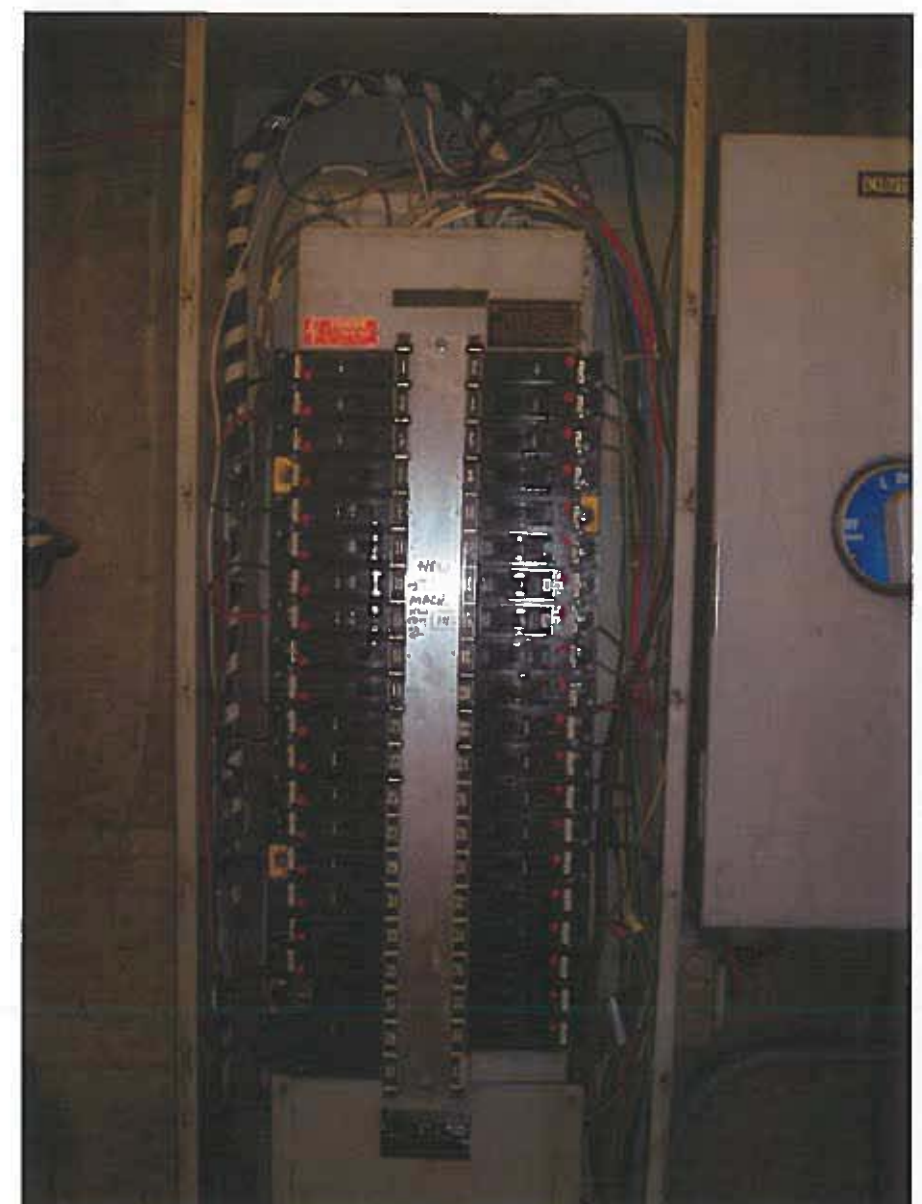
EXISTING PANEL "MNCC"
