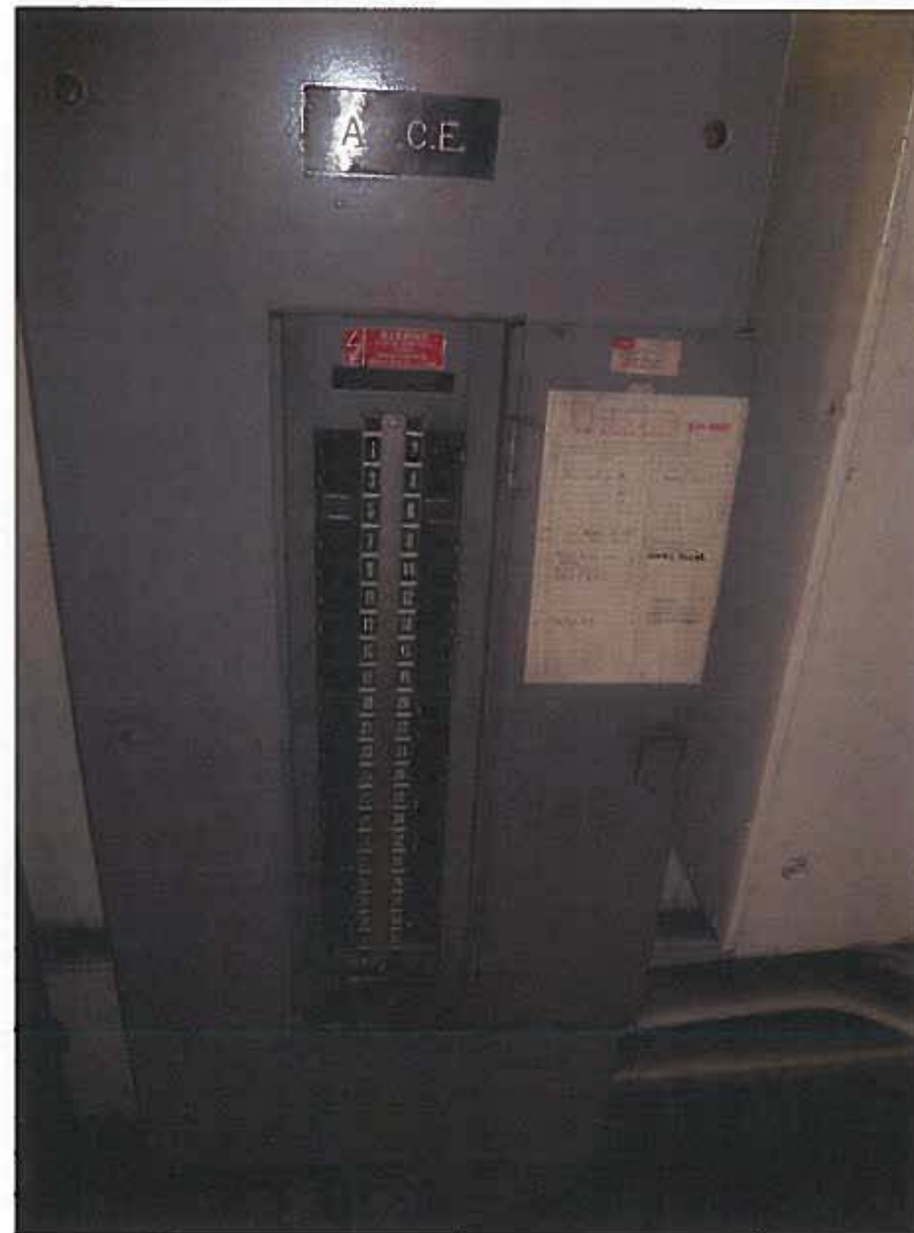
EXISTING PANEL "AFCE"
