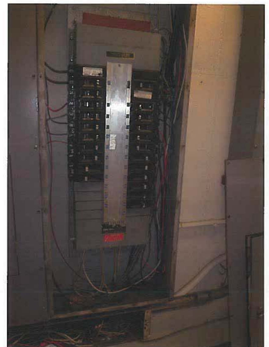
EXISTING PANEL "F-2"
