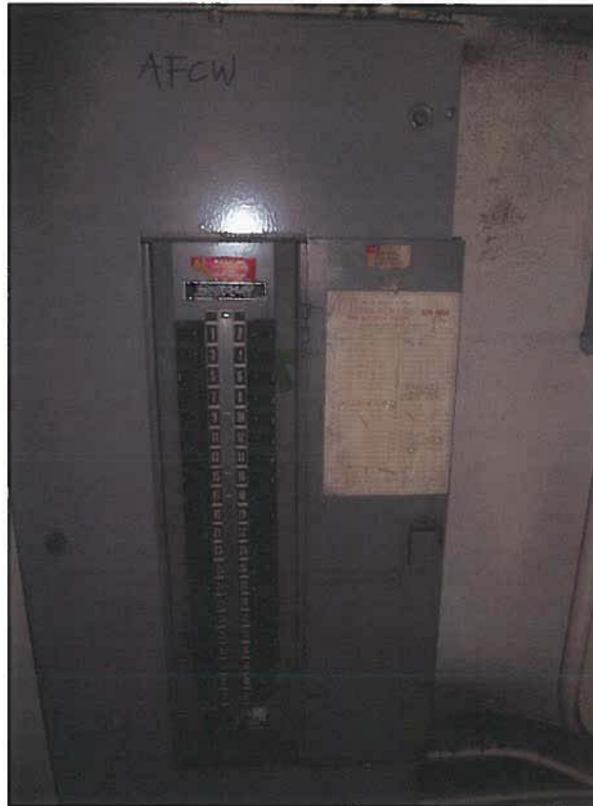
EXISTING PANEL "AFCW"
