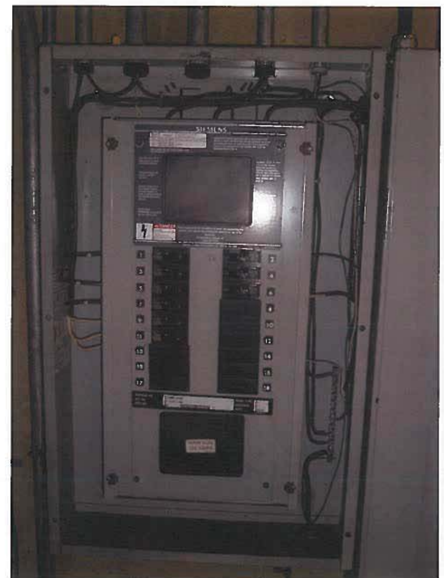
EXISTING PANEL "F1"
