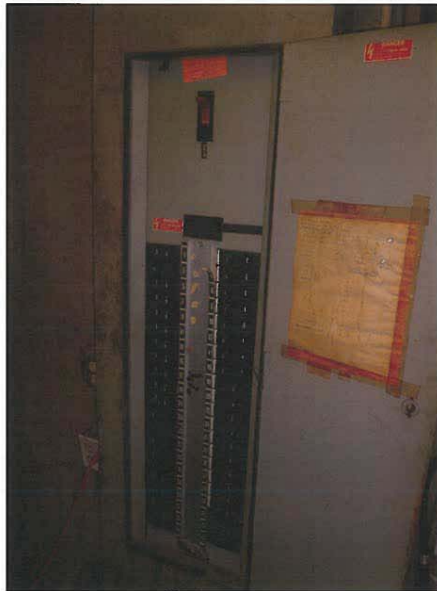
EXISTING PANEL "SF"
