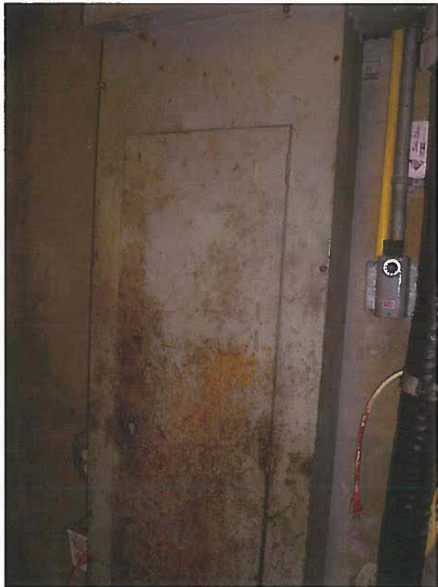
EXISTING PANEL "SF"
