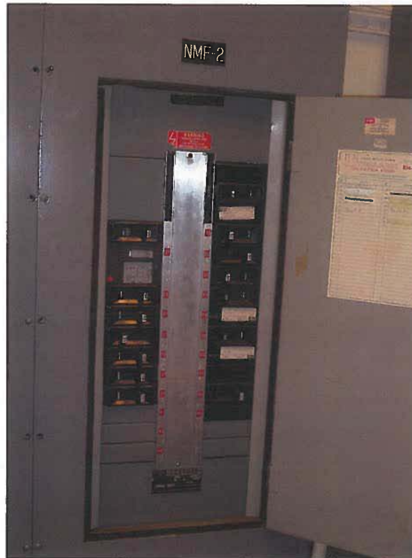
EXISTING PANEL "NMF-2"
