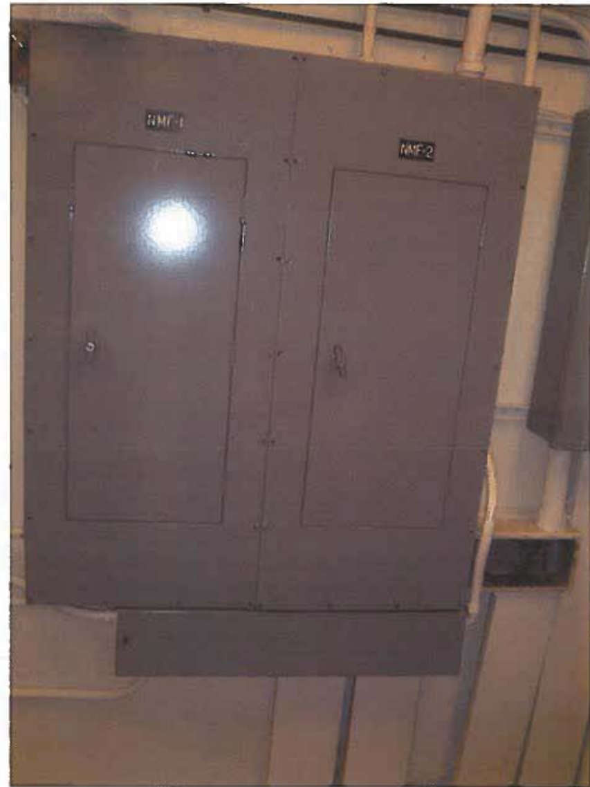
EXISTING PANEL "NMF-2"
